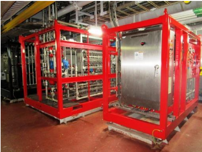
BOP Control Room.
