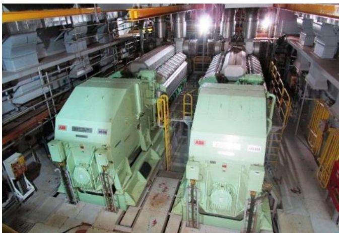
General View of DRU #01 – ARPOADOR generator room
