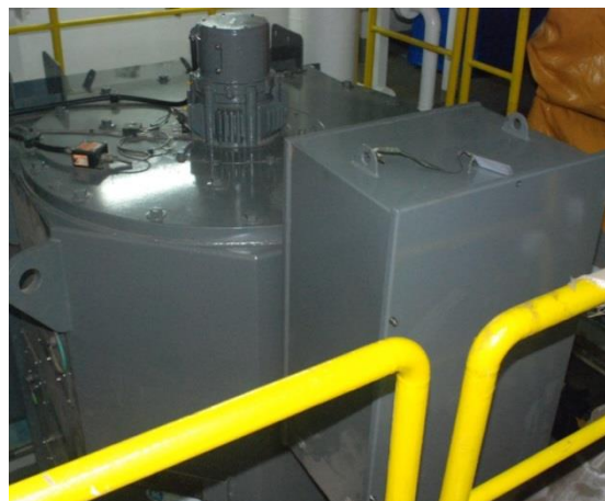
Thruster Electric Engine in FRADE HULL
