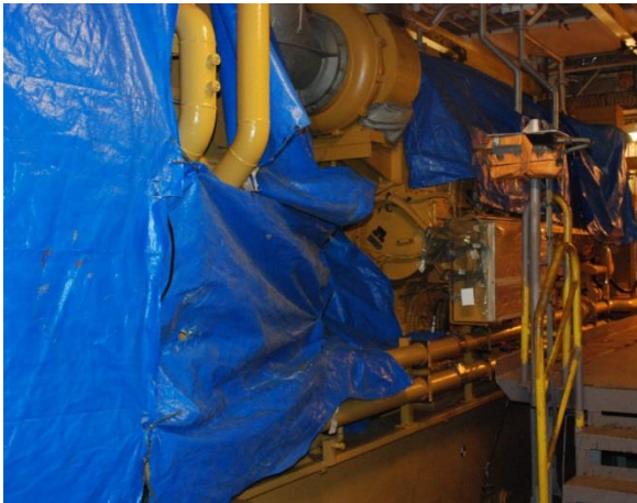
Electric Generators covered with canvas
