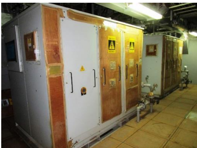
Power transformers energized and identified.
