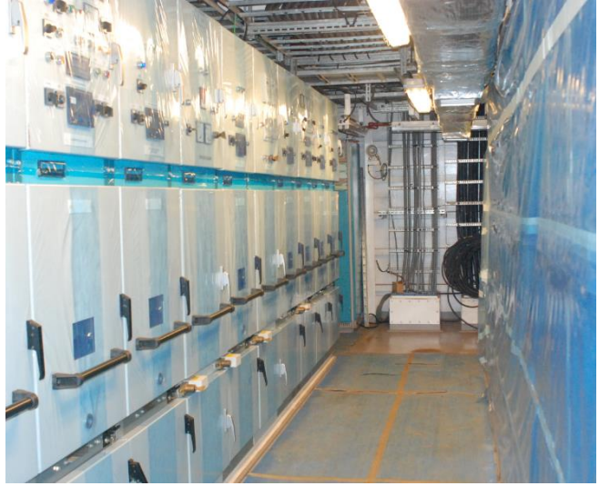
Generator Room - Switchboard
