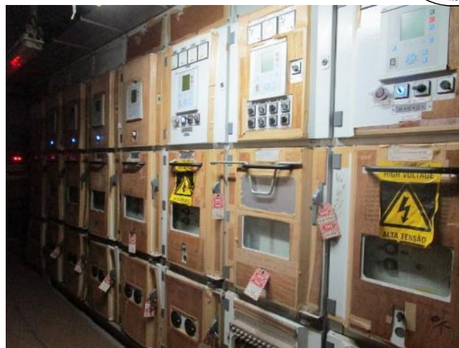
Power transformers energized and identified
