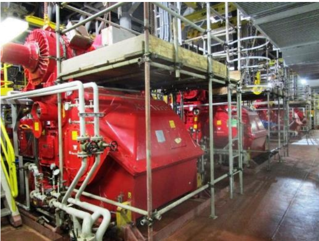
Mud Pumps Room.
